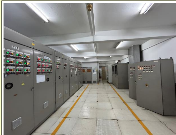
Ruang Control Panel
